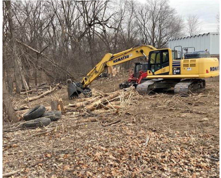
Trees have been removed on the west side of the clubhouse to make way for the underground water pipeline.
